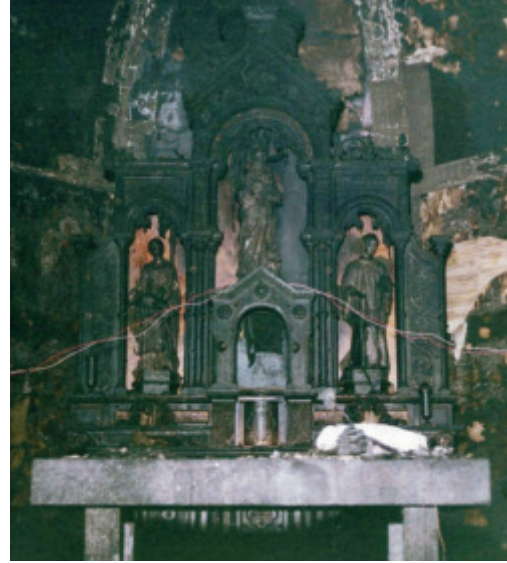
Main altar area inside the church after the fire.
